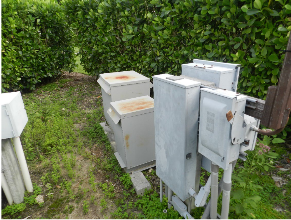
View of electrical panels.
