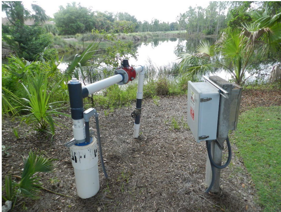
View of irrigation recharge well and associated control panel.
