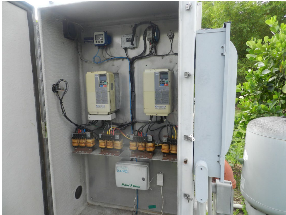
View of irrigation control panels and associated equipment.
